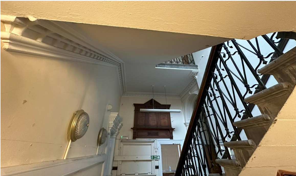
Figure 5: Ground floor stairwell, showing need for decorative and electrical works.
