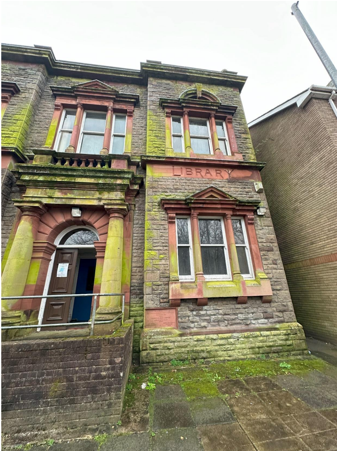
Figure 4: Main facade, showing need for external cleaning.
